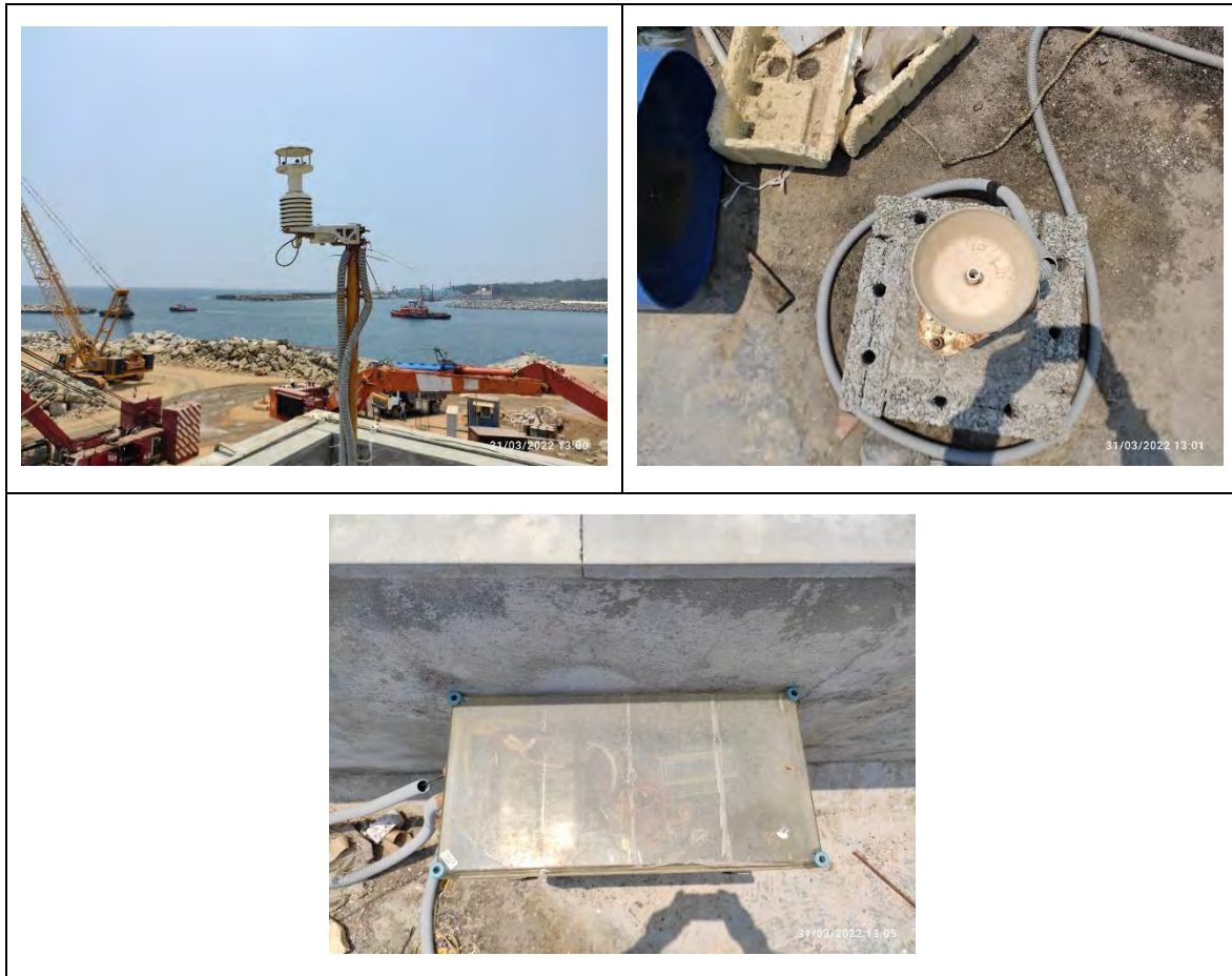
Figure 5-7: AWS on top of Port Control Office building
