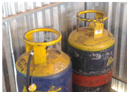
Cooking gas provided in the kitchen of M/s B&R
